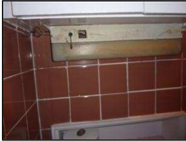
2.4 Picture 2 Obsolete light in bathroom
