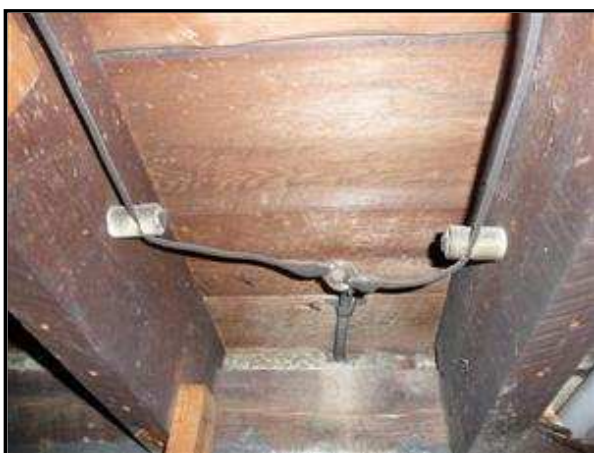
2.2 Picture 3 Knob & tube wiring in basement
