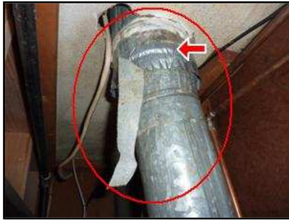
1.4 Picture 4 Duck tape on exhaust flue
