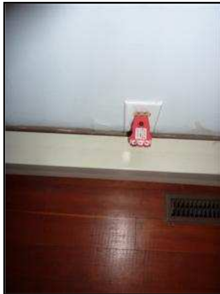
2.4 Picture 1 Dining room: not grounded
