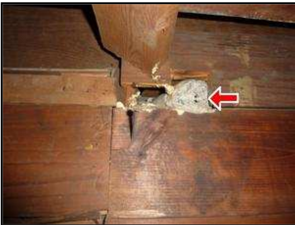
1.4 Picture 2 Possible asbestos
