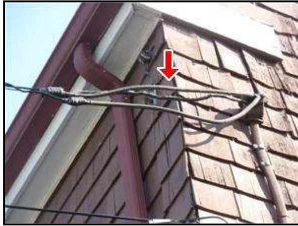
2.0 Picture 1 Wires being pulled off house
