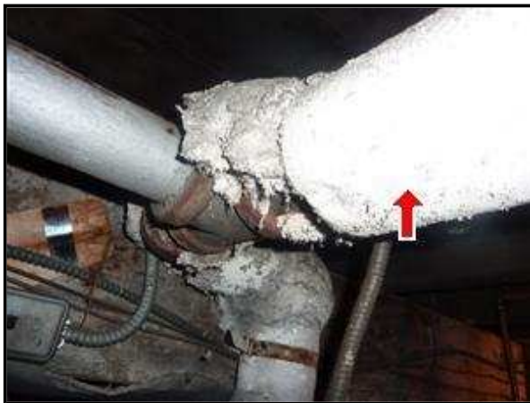
1.4 Picture 3 Frayed pipe insulation
