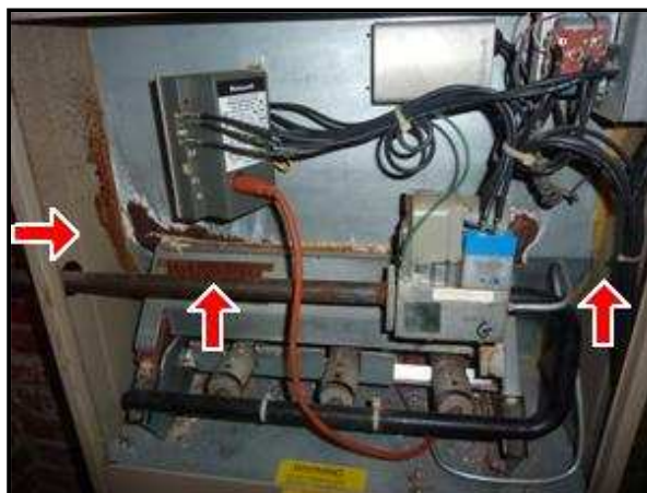
1.0 Picture 1 Rust under cover of furnace
